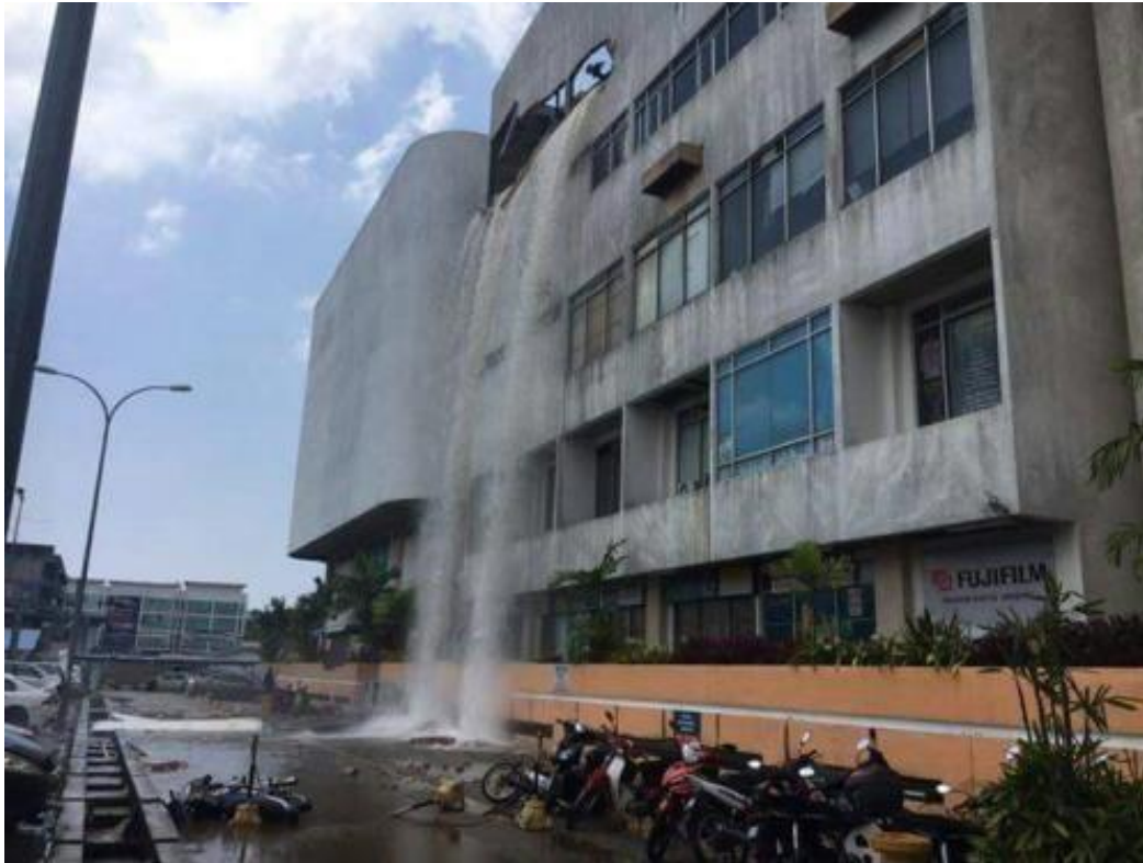
Burst water tank in a 4 storey shopping mall in Kuantan in 2017
