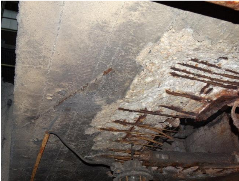
Spalling of concrete with corroded rebars 10
